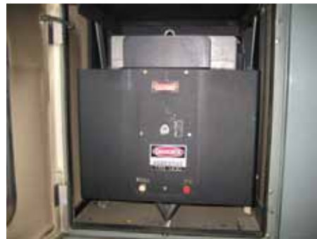
Figure 5.1: Obsolete Westinghouse LA50 ACB
