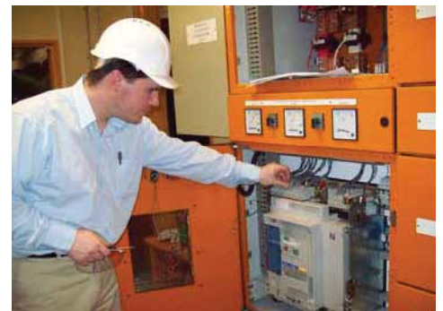
Figure 4.1: Service engineer inspecting an ACB.
