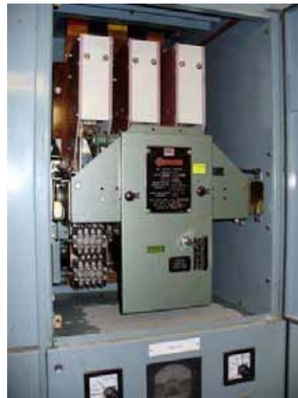
Figure 5.0: Obsolete NILSEN ACB
