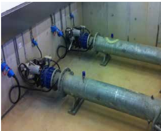
Figure 3: Water Pump Station
